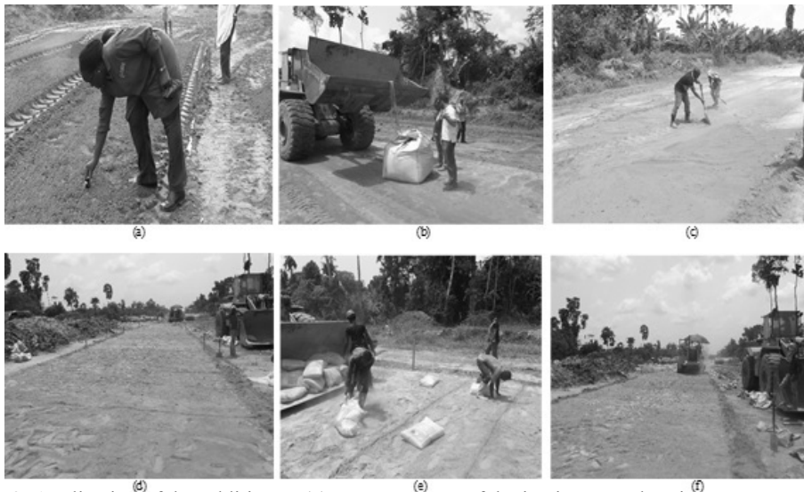
Plate 2: Application of dry additives – (a): Measurement of the in-situ natural moisture content; (b): DCA brought in jute-bag; (c): Manual spreading of additives on scarified section; (d): All the additives applied on the subgrade; (e): Laying of bags of cement within grids; (f): Cement added on top of the additives
