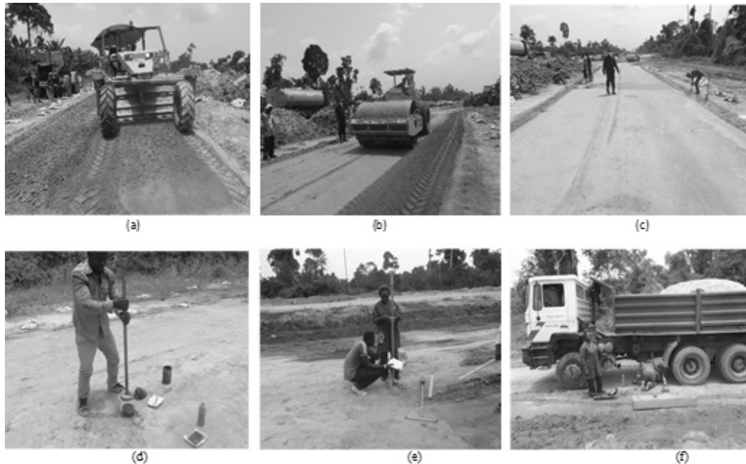
Plate 3: Mixing and Compaction – (a): In-situ mixing of soil, additives and cement by the rake mixer; (b): Compaction using vibrating steel-drum roller; (c): Stabilised subgrade; (d): Mauually coring of stabilised soil; (e): DCP testing of section; (f): Field plate loading test
