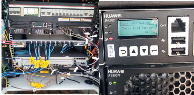
Figure 4:GLO Cabinet Base Band unit.
